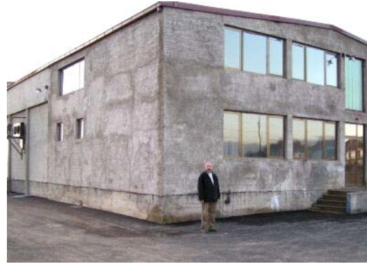
New meat processing factory is situated very close to the strategic highway "Corridor 10", which connects Central Europe and Greece
